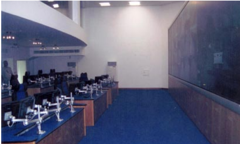
Control center C4i for coastal surveillance in Kuwait
